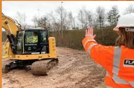
People Plant Interface top fatal injury in construction
